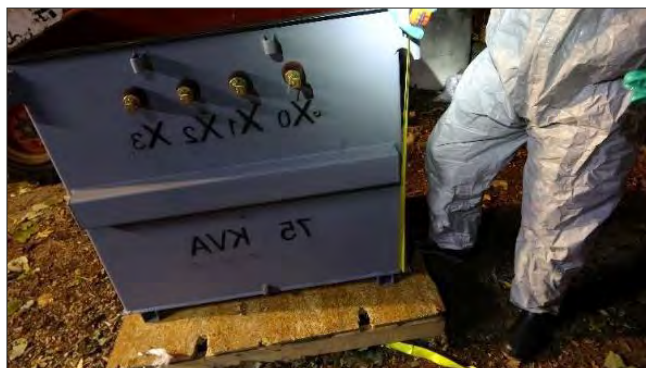
Figure 48. Electric Transformer Seized by Atlanta Field Division
